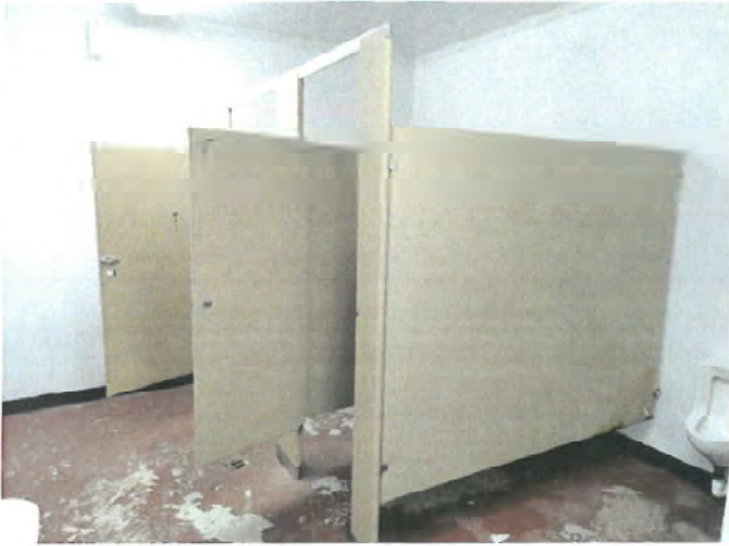
Restrooms- Degraded flooring and walls, damaged stalls, inadequate urinal and toilet facilities
