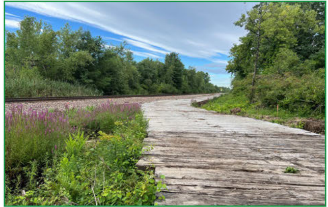
The clearing of land adjacent to the train tracks is to make room for the CHPE power line.
